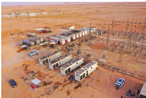
Fig. 2 The power system plant in Rutba city.
