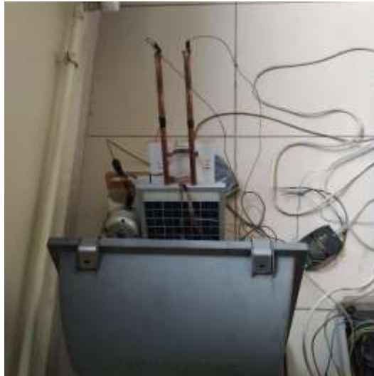
Fig. 9. Heat pipe condition
