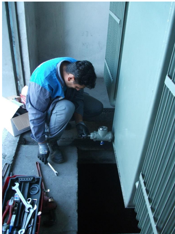
Fig. 1 Taking Oil Samples from Transformers
