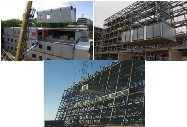
Figure 2. A Composite module [17]. B. Steel core modules C. Schemes with outer frame
