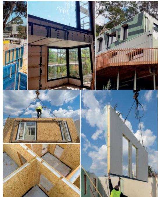
Fig 1. A.B.C. Modular structures; source: Chris Neylon/CarbonLite; D.E.F. Prefab methods; source: Bilanol/iStockPhoto, brizmaker/iStockPhoto, brizmaker/iStockPhoto
