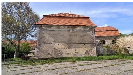
Fig 1 View of one wall of the fortress from which we will create a 3D model. This is the wall of a brick building that served the army until a few years ago.
